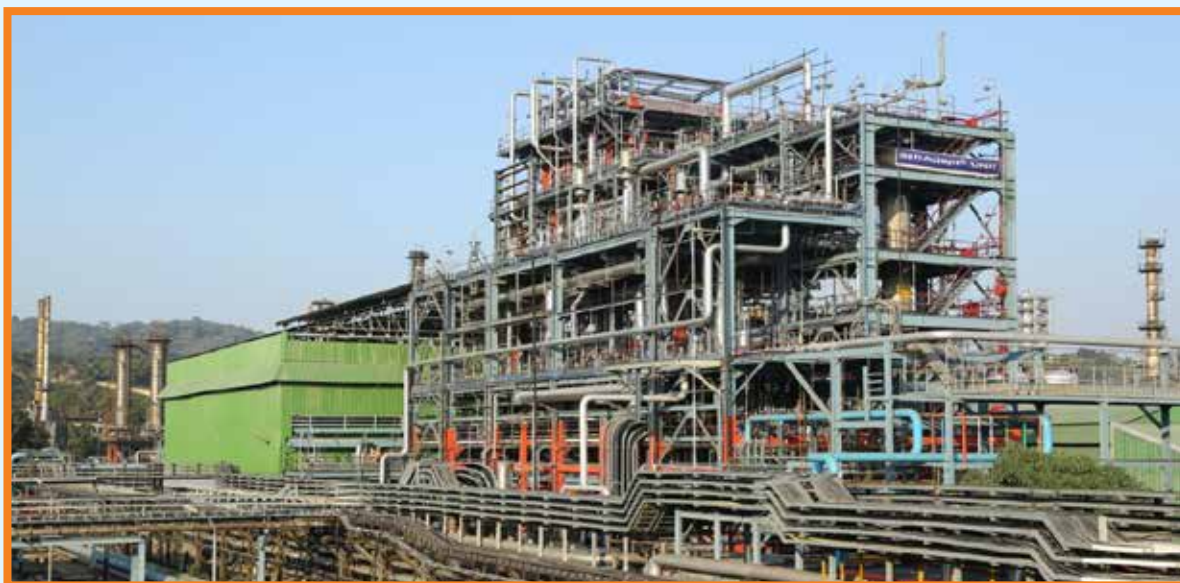
INDAdeptG Unit at Guwahati Refinery
